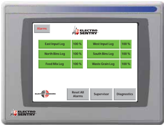
Normal Operation "Home" Screen View — No Alarms
