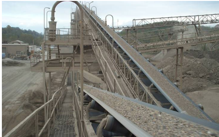
Typical Overland Conveyor Setup in a Rock Quarry
