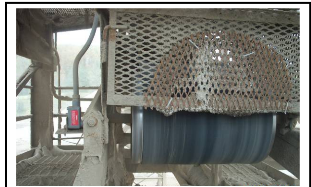
Monitoring the Tail Pulley on a Conveyor
