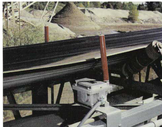
Typical Belt Alignment Switch Installation
