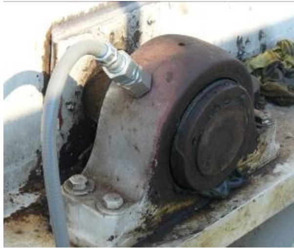
TT420-Z (DI) Temperature Probe mounted on a bearing
